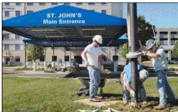
Construction workers from DeWitt and Associates relocate a flag pole to the temporary entrance at St John's Hospital. A flurry of activity was taking place to get the entrance ready for today.
